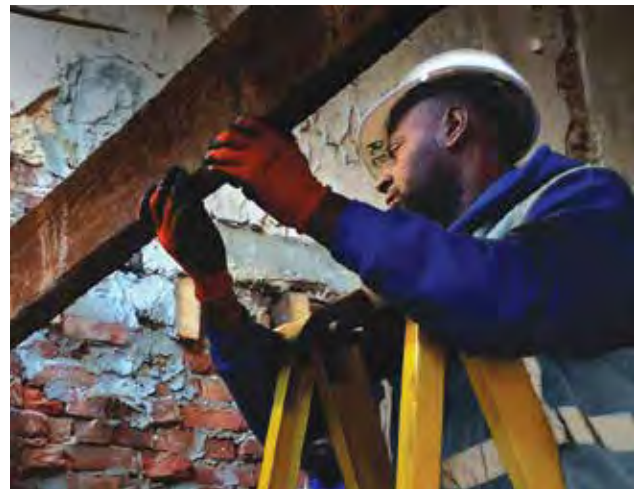
Humanim deconstructs abandoned homes and recovers material for further processing or reuse by architects, furniture makers, artisans and builders.
